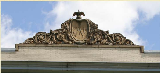
The building is crowned by a prominent cornice. Once, the words École normale were engraved above.
